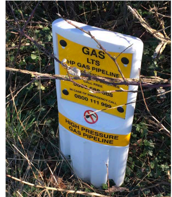
Gas pipeline marker
