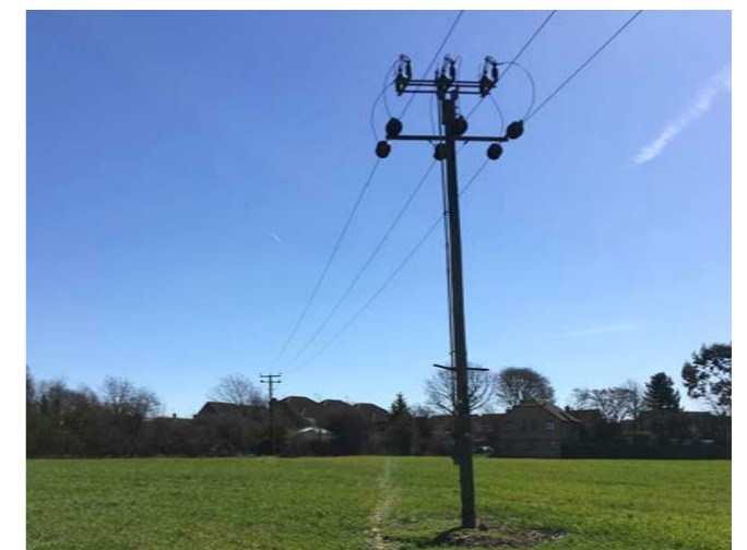
Overhead power lines
